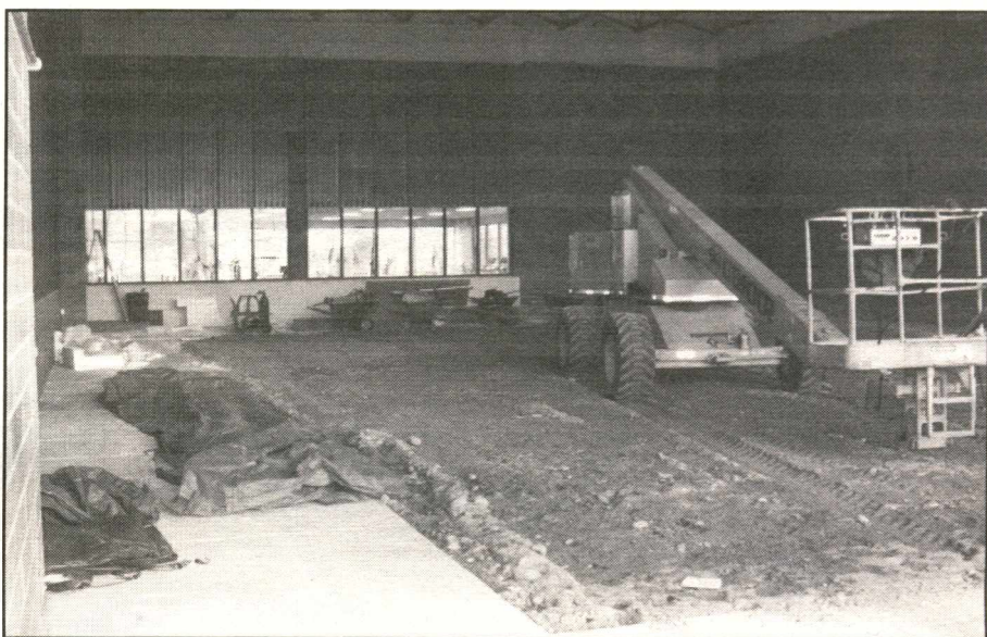
The remains of what used to be NNU's indoor pool, now being prepped for conversion to an indoor soccer field (photo by Robin McConkey).
