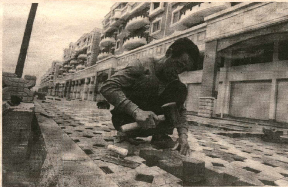
A construction worker works on a residential development built by Taiwanese developers in Xiamen, China February 19. Xiamen is a great example of why Chinese leaders will think twice before attacking the island they consider their renegade province: Taiwanese companies have invested so heavily in this city that their enterprises are the backbone of its economy. Xiamen is only 2.5 kilometers from the closest island of Taiwan.
