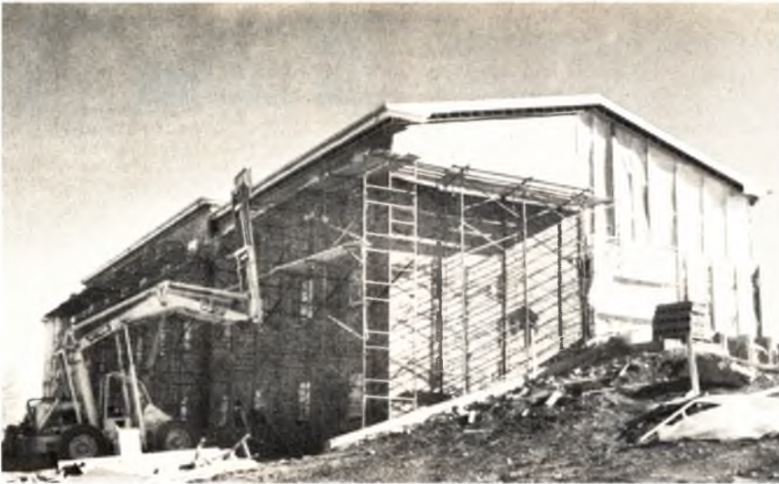
A new residence hall for women, project of the "No Room in the Inn" campaign, is under construction. It will house 125 women and will be ready for occupancy for the 1981 fall term.
