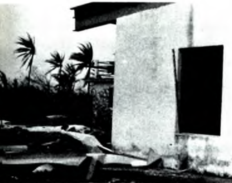
Photo of part of the church after "Pamela" passed by. On the back of the picture Rev. Rich wrote: "Window blown out—end of roof off. This is part of our backyard. Water stains everywhere!"
