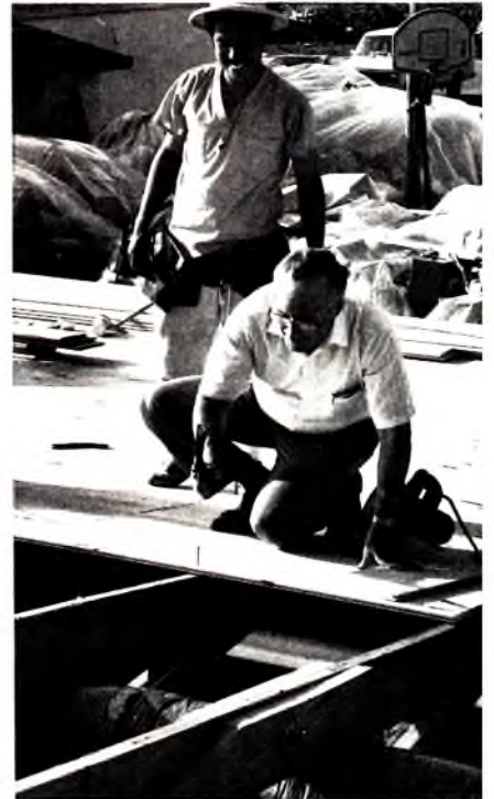
General Superintendent Donald D. Owens joins in the rebuilding effort in Southern Florida. During his visit to the area, he helped put a new roof on the fellowship hall of the Good Samaritan Church of the Nazarene.
