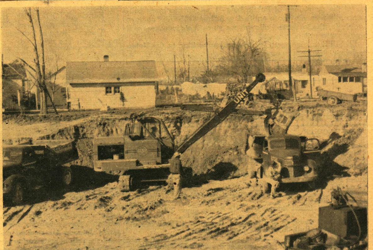
View of "The Hole" on the corner of Juniper and Dewey as seen late last week. The earth moving equipment of all descriptions, including bulldozers and power shovels, worked at full speed in the first step toward building the new 108x140-foot College Church building.
